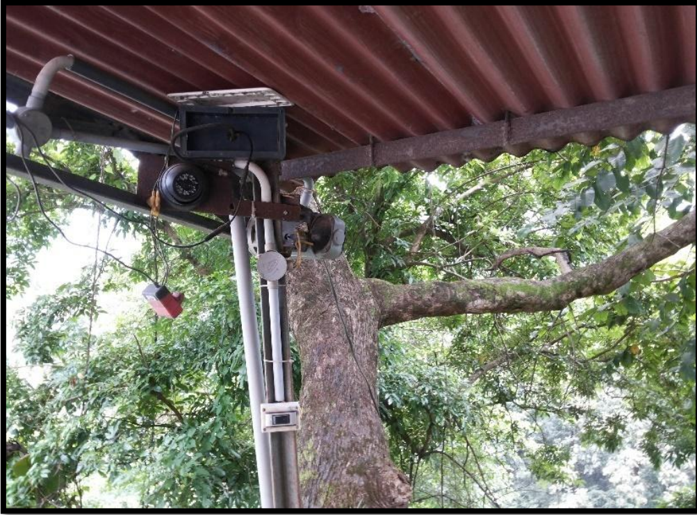
Warning alarm installed in the project site
