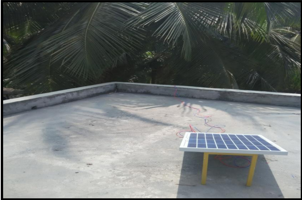
Solar panel installed in project site
