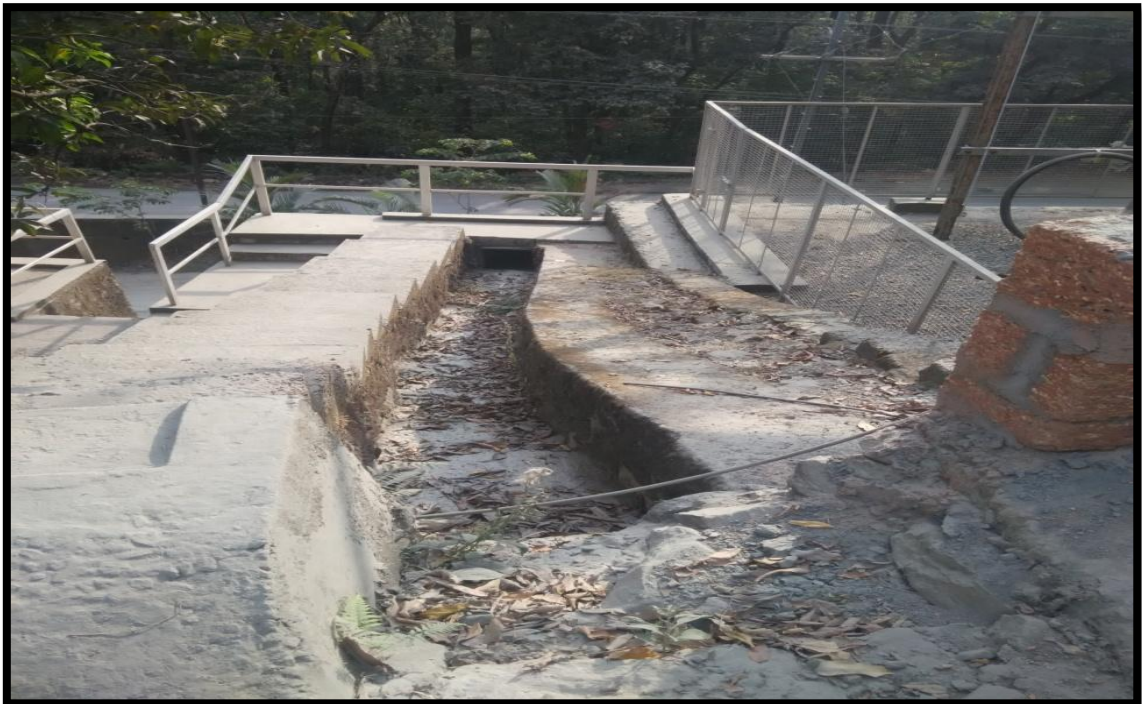
Garland drains for storm water management
